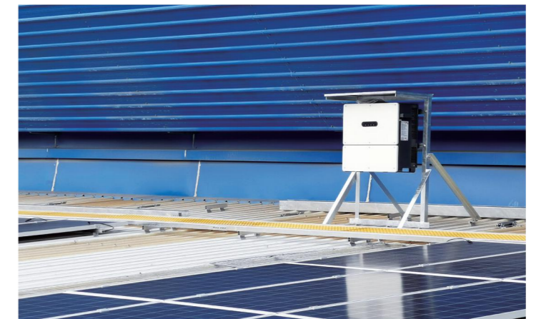
12MW Dalian Roof-top PV Project in China
