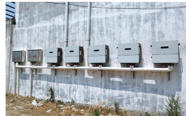
Rooftop PV Project in Shandong
