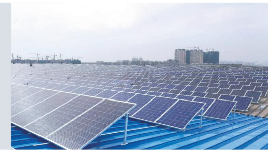
Street-usage PV Station Lingyang, Ju county, Rizhao City, Shandong Province
