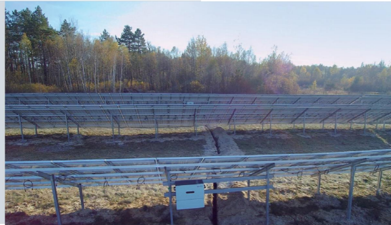
Ukraine 15MW Solar Plant
