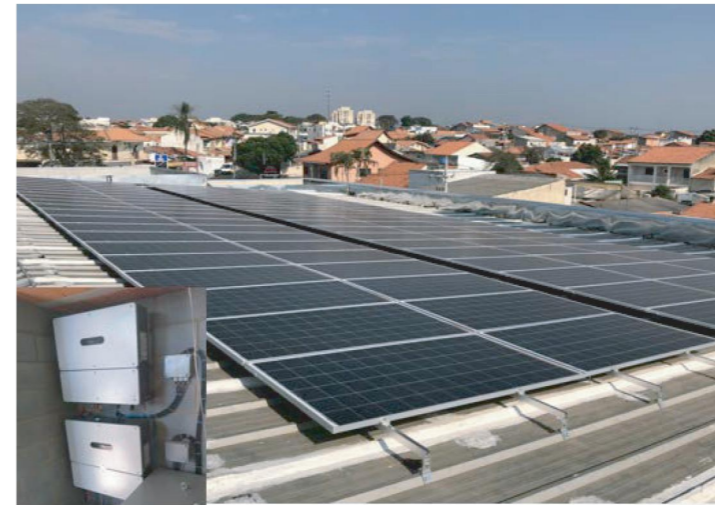
Brazil 500kW Rooftop Project
