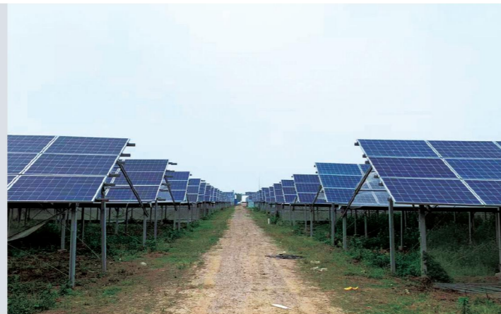
Solar Renewable Project in Anqiu
