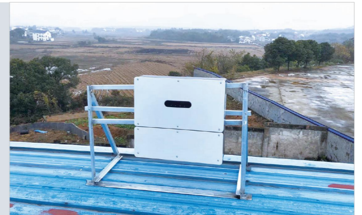
Roof-top PV Project in Hunan China
